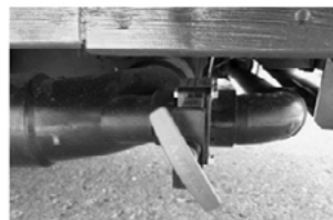
Black/Grey Tank Drain and Valve
