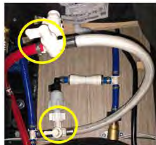
Water heater Bypass Access shown in NORMAL mode
