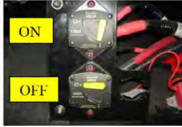
Breakers at rear of coach
